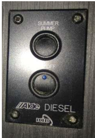
Additional switches for Diesel Alde.
